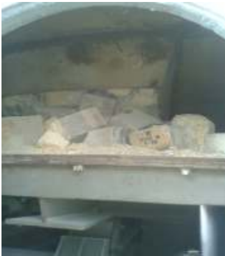
Fig-2: Brick collapsed from kiln
